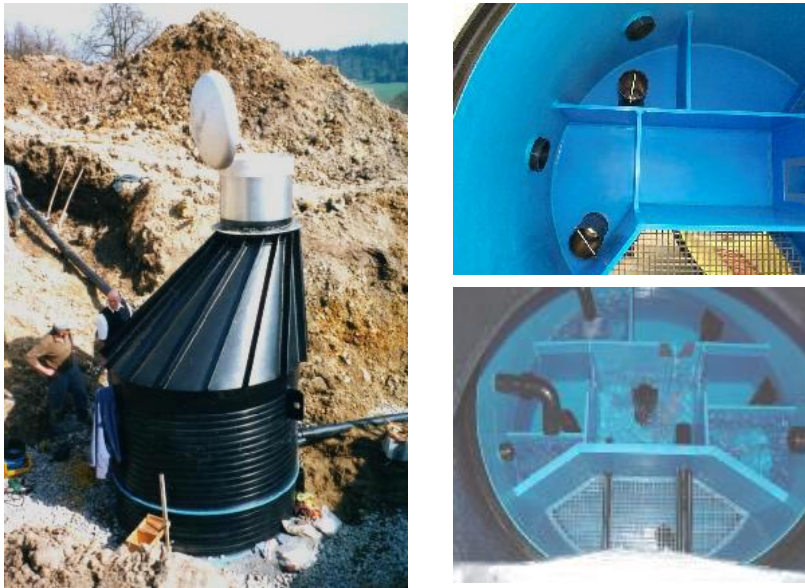
Figure 6: left: collecting shaft with a conical entrance; right: the inside of collecting shafts
