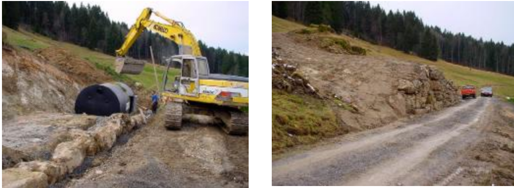
Figure 9: installation of a storage tank: ID 1800 mm and a volume about 10 m 3
